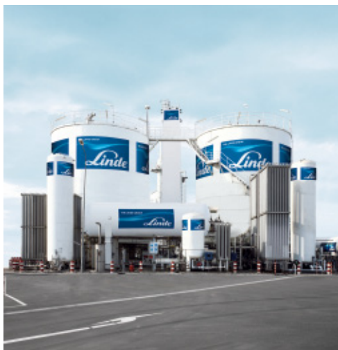
Figure 4: Cryogenic air separation plant
