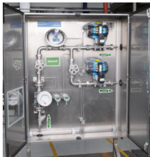
Figure 16: Complex measuring and metering station for nitrogen intended for the inerting of vessels, mixers and reactors [4]
