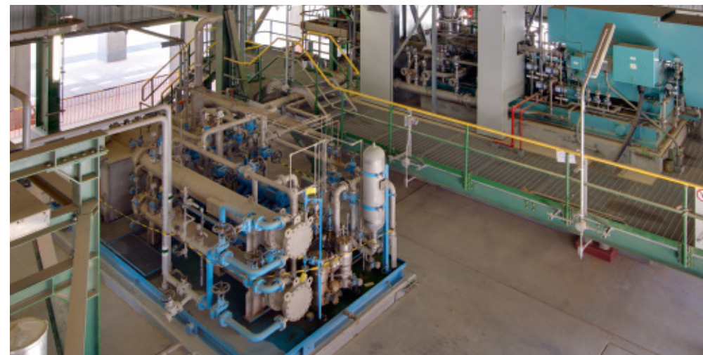
Figure 6: Small membrane separation plant
