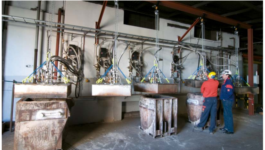
OXYGON® 400 preheating systems installed at SKF in Katrineholm, Sweden; 1 ton ladles are heated in 6 stations.
